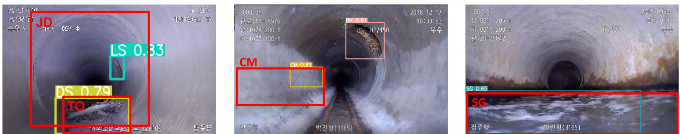
FIGURE 12. Detection results for various types of sewer cracks (Failed cases)
