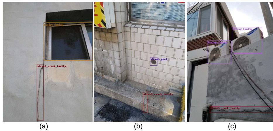
Fig. 9. AD-TR model performance in multidefect scenarios: (a) crack and window faulty; (b) peeling and crack; and (c) crack and falling objects.
